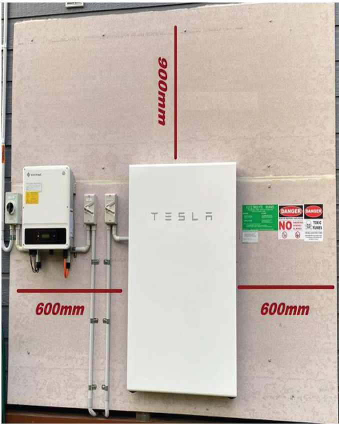
Compliant installation of Cement Sheets
